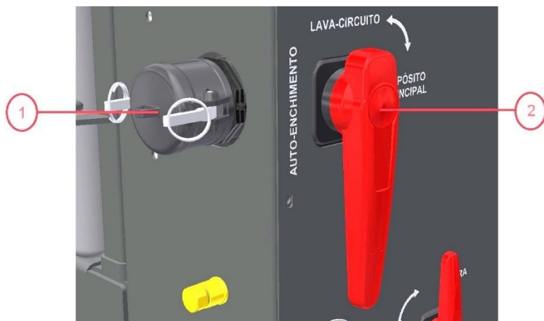
Figure 6.13 – Ex. Panneau de vannes
